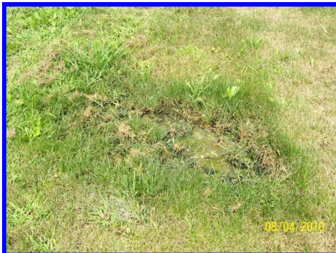
Picture shows raw sewage at the ground surface from failing septic system from 10/20/2009 investigation. This system was repaired in the fall of 2010.
