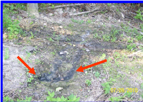
Blackish-grey residue is sewage leaching to the ground surface from the failing septic system.
