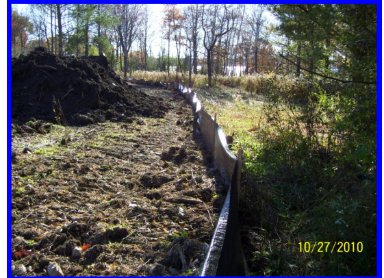
Active construction site within the watershed. Silt fence in place protects sensitive areas and prevents disturbed soil from moving offsite.
