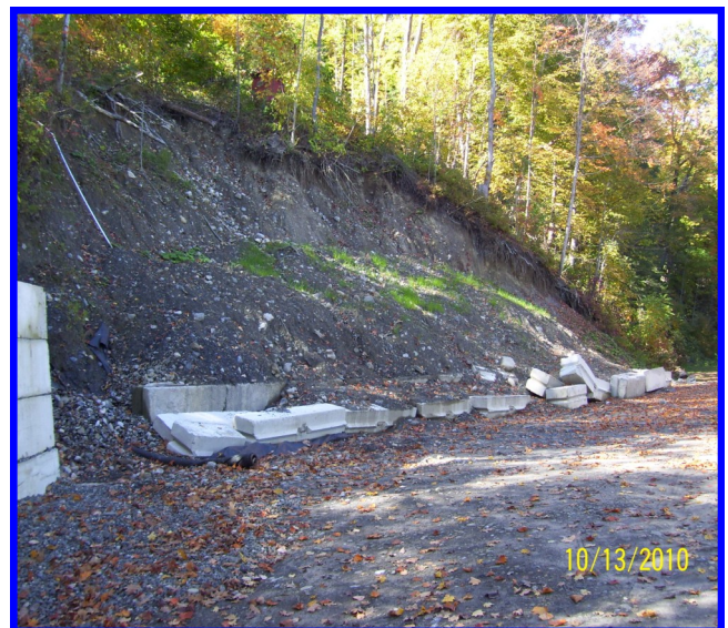
Picture shows failed wall at lakefront property. Wall failed due to poor construction and upslope drainage issues not being addressed.
