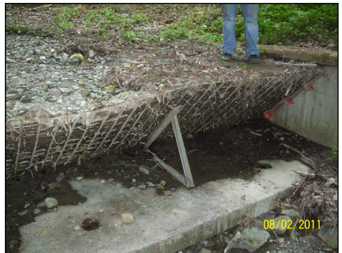
Assistant watershed inspector Sandro Valle stands atop the filled-in trash grate
