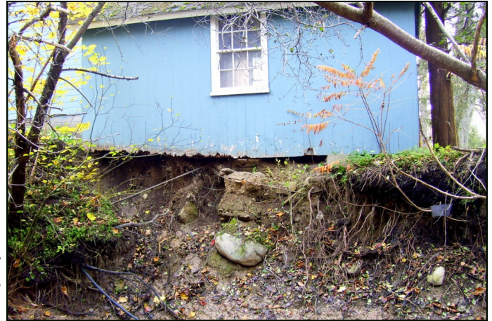
The photo to the right demonstrates how the bank is undermining the shed sitting directly above. As high flow due to heavy rain events gush through a stream corridor, it carries with it sediment from the banks of the stream sometimes resulting in severe erosion.
